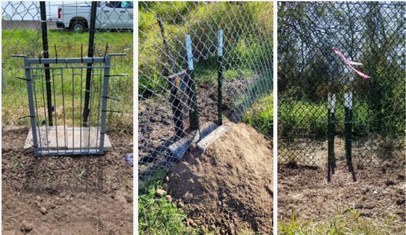
Figure 3-36 Experimental escape chute design alternatives installed in a highway wildlife exclusion fence. This device was designed for ocelots in Texas (photo credits: John Young, TxDOT).
