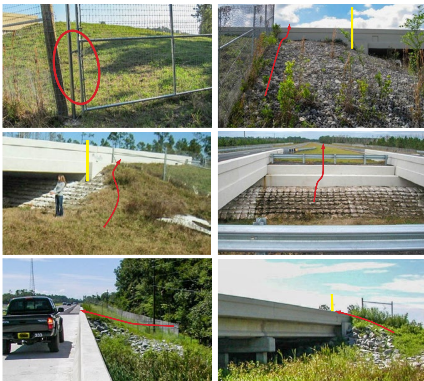
Figure 3-33 Examples of fence gaps that potentially allow wildlife to access the road. End posts need to be placed directly against the structure and the fence needs to be continuous across corner and median gaps where animals can traverse slopes and hop over short barrier walls.
