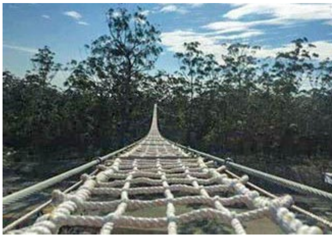
Figure 3-45 A canopy rope bridge installed over a roadway in Australia. Photo source: Fauna Crossings: Kempsey to Kundabung in NSW Fauna Crossings .
