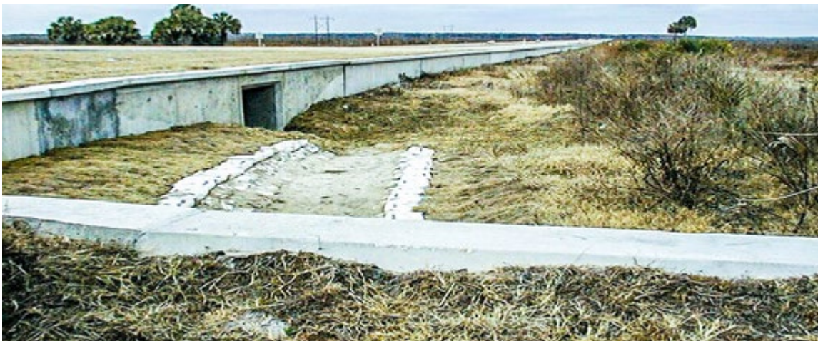
Figure 3-29 An image of the Paynes Prairie State Preserve herpetofauna barrier wall on US 441. On average the wall is 4 ft above grade and includes an overhanging lip to help prevent climbing.
