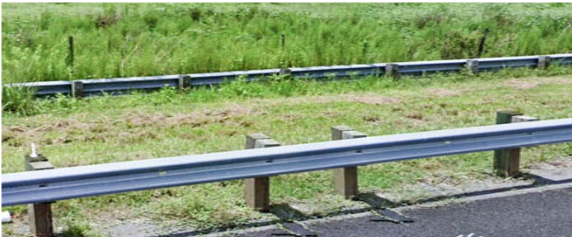
Figure 3-30 Installation of thrie-beam guardrail (in the background) used as a barrier to prevent trespass by small mammals and herpetofauna in Paynes Prairie State Preserve.
